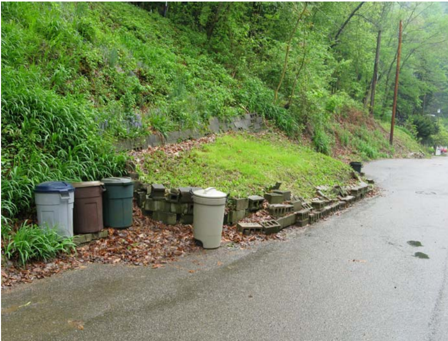
Slate Street slump – note how it has covered a part of the road
