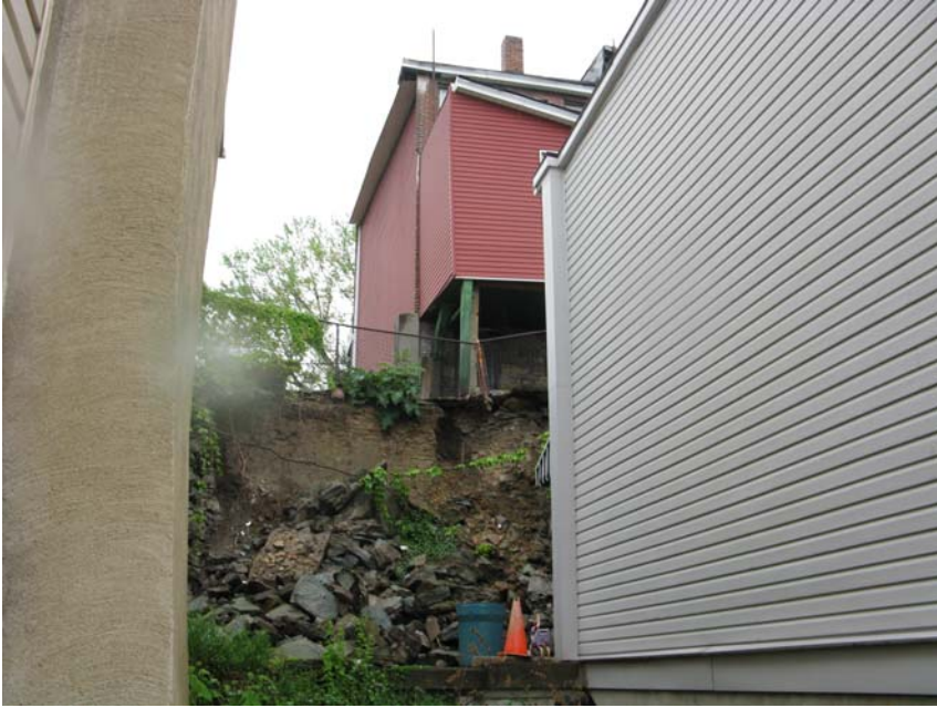
Flowers Avenue Wall – building on a retaining wall can lead to the failure of the wall and the hillside, resulting in serious damage to buildings and properties above and below the hill.
